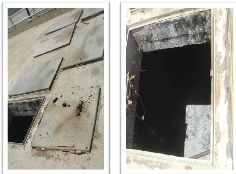
Figure 5.4 - Pumping stations “in situ”; source: Aqualogy Aqua Ambiente
