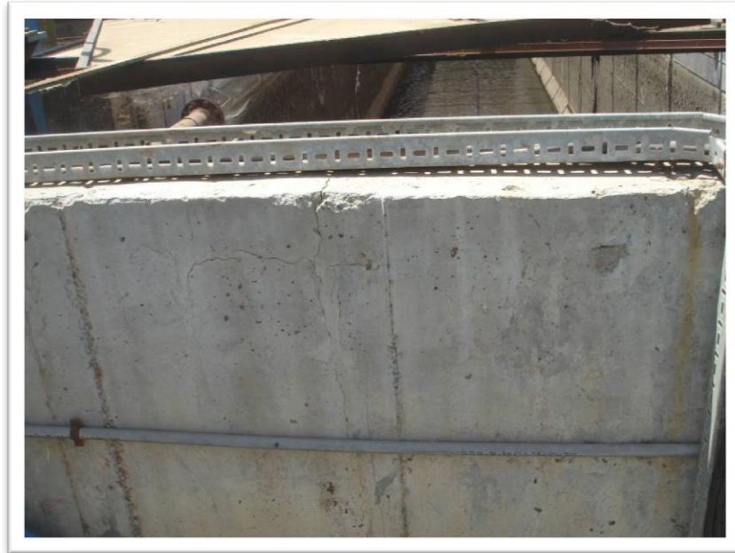
Figure 5.13 - Pathologies in concrete by source: Aqualogy Aqua Ambiente
