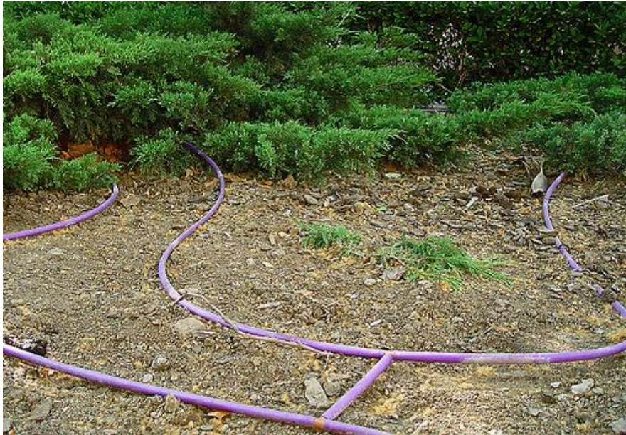
Figure 9.4 - Reclaimed water pipe in the irrigation area; source: Aqualogy Aqua Ambiente
