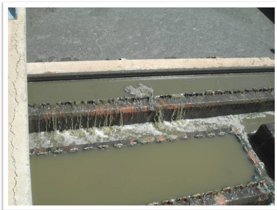
Figure 5.10 - Water outflow of the primary decanter by source: Aqualogy Aqua Ambiente
