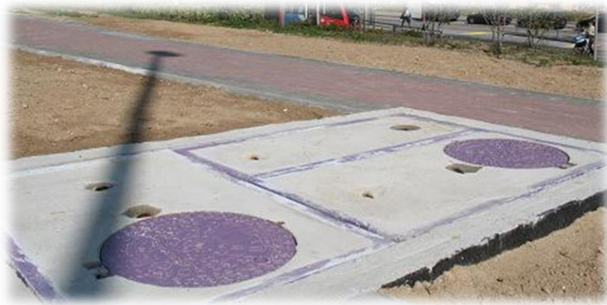
Figure 9.1 - Manhole covers of reclaimed water; source: Aqualogy Aqua Ambiente
