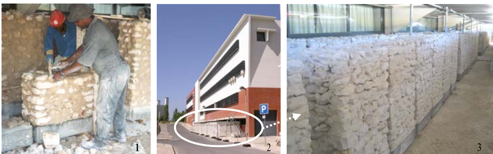
1 – construction of the experimental models, using traditional techniques; 2 – curing place of the models; 3 – inside of the curing place
