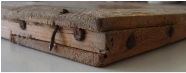
Figure 19: Corner detail: simple mortise & tenon with square corners. Protruding nail is evident.
