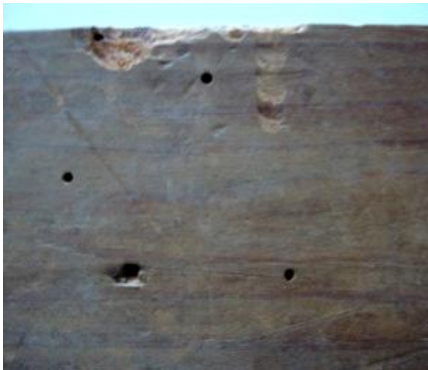
Figure 20: Exit holes from wood boring insects: small circular holes distributed randomly.
