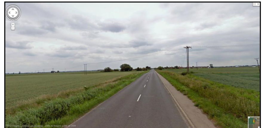
Appendix Figure III.4 - 200 ACSR OHL with pole 73 on the right and pole 74 on the left.
