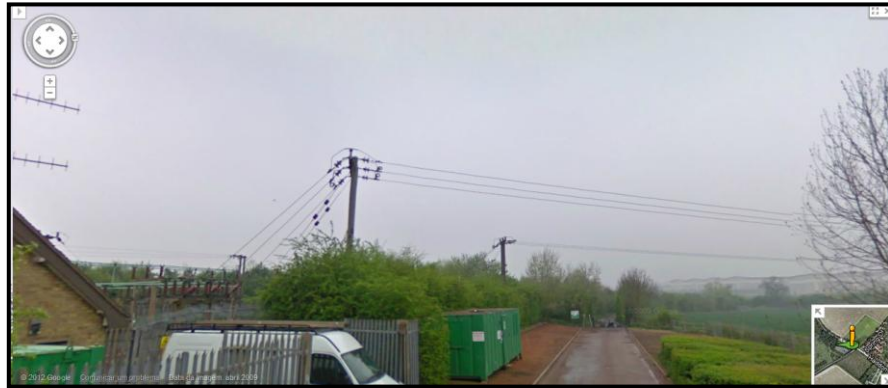
Appendix Figure IV.1 - 150 ACSR OHL coming out of Frct Primary Substation.
