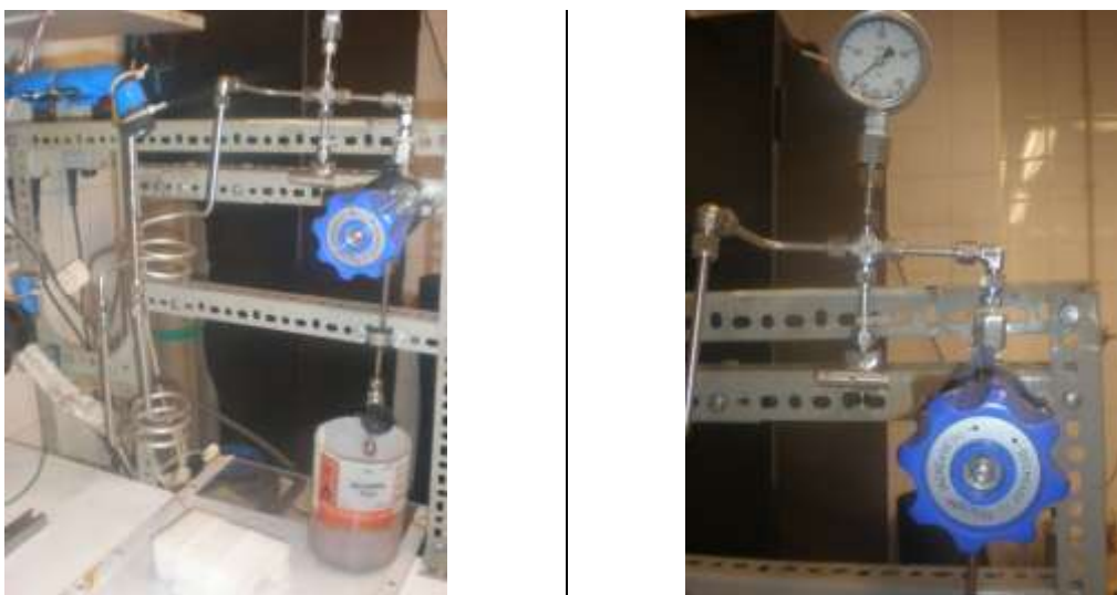
Figure 2.1.8: Separation section. BPR Valve
