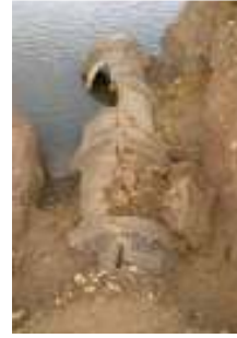
Figure 2. Crack observed at the bottom outlet of Herdade da Misericórdia dam (2006).
