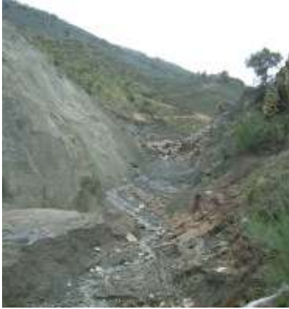
Figure 15. Dam breach, view from downstream. The rock formation from the riverbed is visible.
