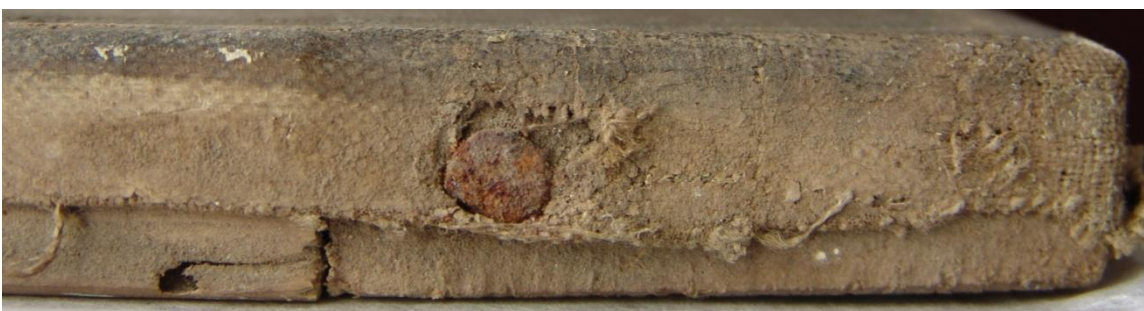
Fig.IV.4. Normal light photographic detail of rusted tack at the top of the right tacking margin of the painting.
