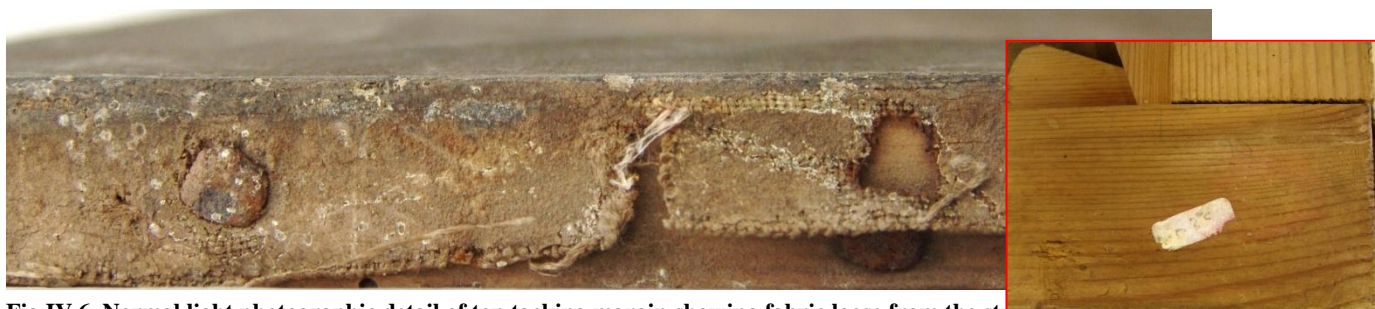
Fig.IV.6. Normal light photographic detail of top tacking margin showing fabric loose from the stretcher.
