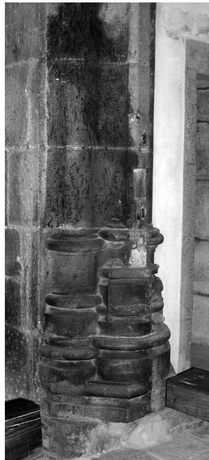
Figure 4. Green biofilm covering the granite surface of chapel 3 left column.
