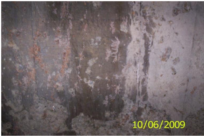
Figure 5 Discolouration of concrete surface
