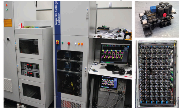
(b) Converter in its cabinet (left), one full-bridge SM (top-right) and the 6 stacks of series-connected SMs with the DS at the bottom (bottom-right).
