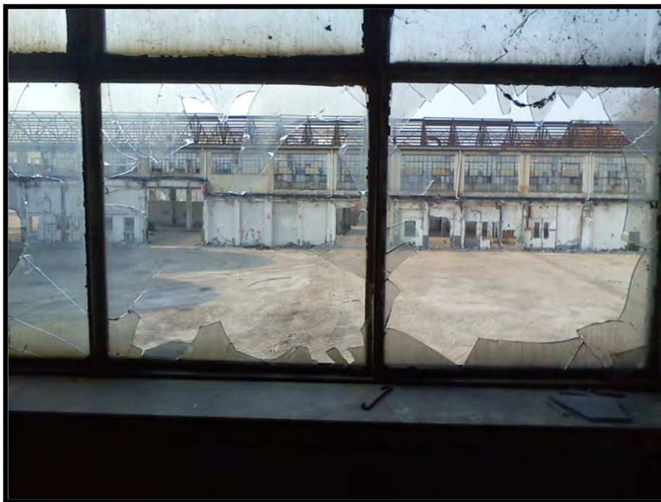
'The Hotel', Turin. View of the courtyard from the inside Photo- Daniel Senovilla, 2011
