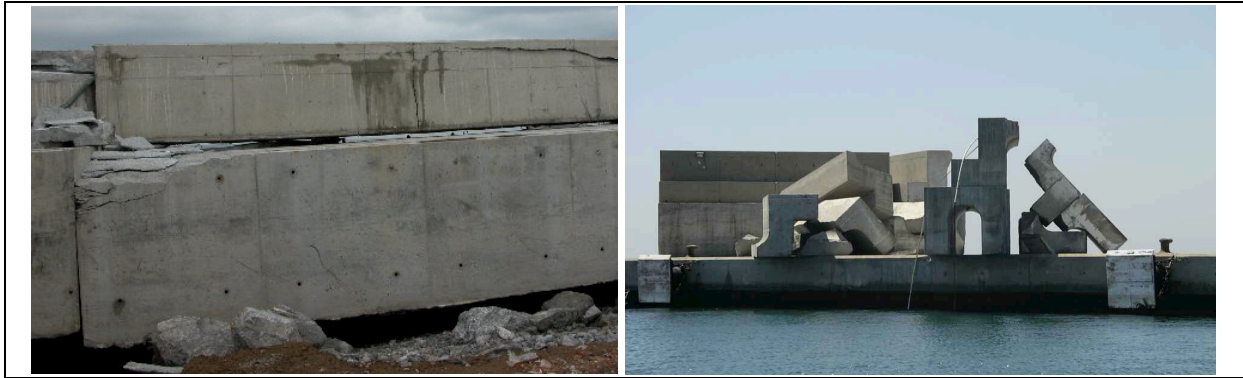
Figure 6: Problems in bulky mass concrete elements: cracking in Ferrol Prioriño Cape Harbour 2001 (left) and collapse in Motril Harbour 2004 (right)
