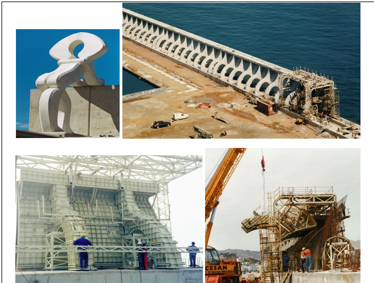
Figure 8: Port of Tazacorte beacon (up, left) and formwork in Málaga “gothic crown wall”
