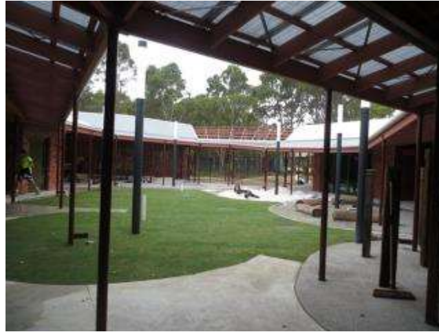
Figure 42: Middle Swan Children and Family Centre - Courtyard area under construction (Source: Formworks Architecture 2013).
