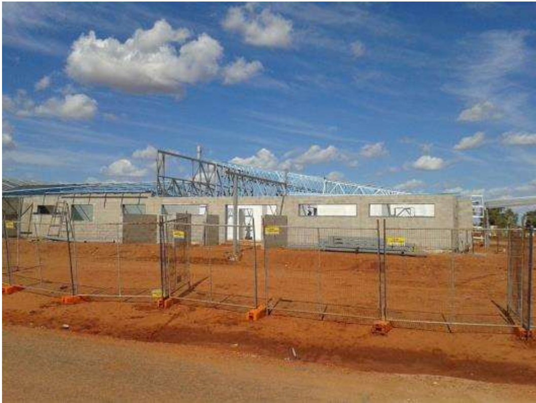
Figure 54: Kurdu Kurdu Kurlangu Child and Family Centre. Centre under construction in January 2014 (Yuendumu Community 2014).
