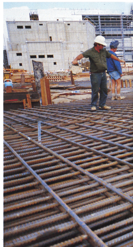
Top right: Early construction on the main support columns of a cooling tower.
