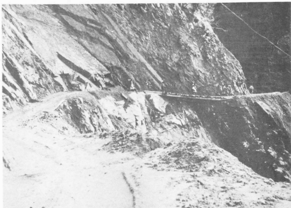
Plate 9. The Steele Falls section of the new Wau-Bulldog Road under construction where it runs along a cliff face of steeply inclined rock strata, New Guinea, 9 July 1944.
