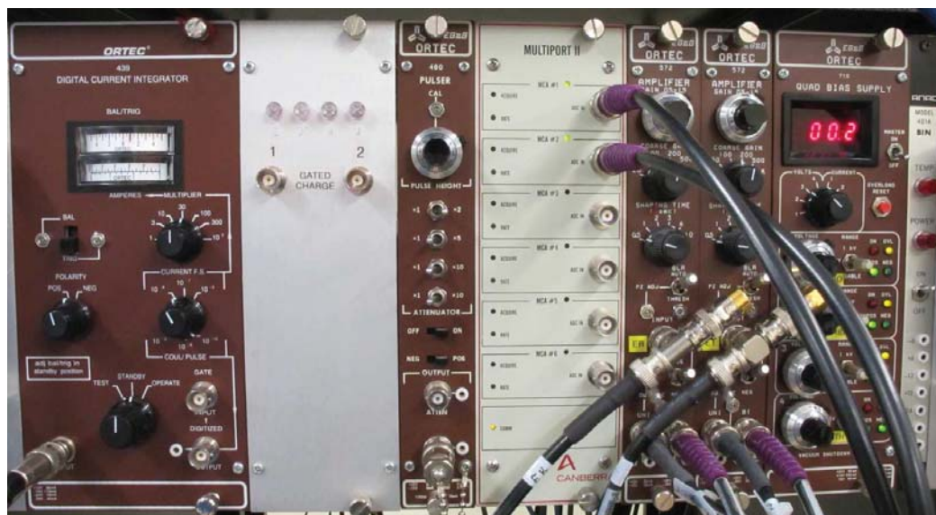
Figure C.25: NIM rack enclosure for beam line 2. From left to right, rack contains digital charge integrator, JTAG communications interface, pulser, Multiport II MCA, 2 amplifiers and a quad port bias supply. The overriding power switch is located on the far right.
