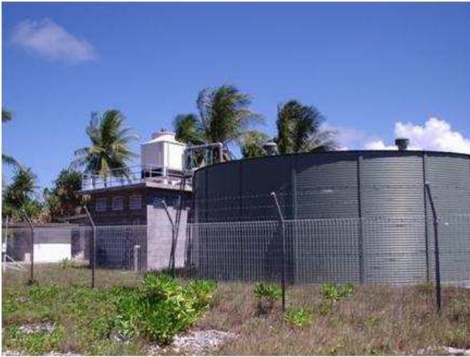
Figure 6-2: Bonriki chlorination plant
