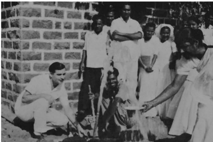
Inauguration new water system at Umri Mission Hospital, India
