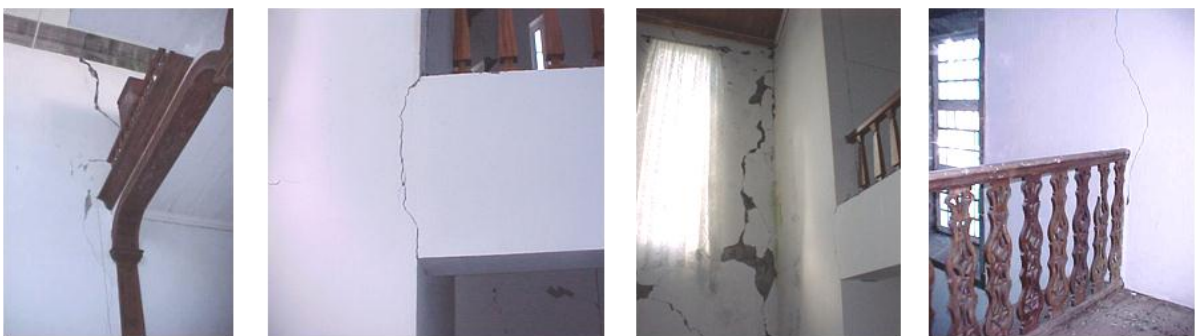
Figure 3. Consequential damages of the interaction between high choir and sidewalls of Azores churches [Costa and Vasconcelos, 1999]
