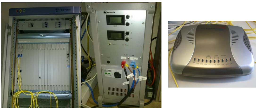
Figure 3.3: (left) OLT-AN5116-02 rack and power supply (right) ONU – AN5006-074
