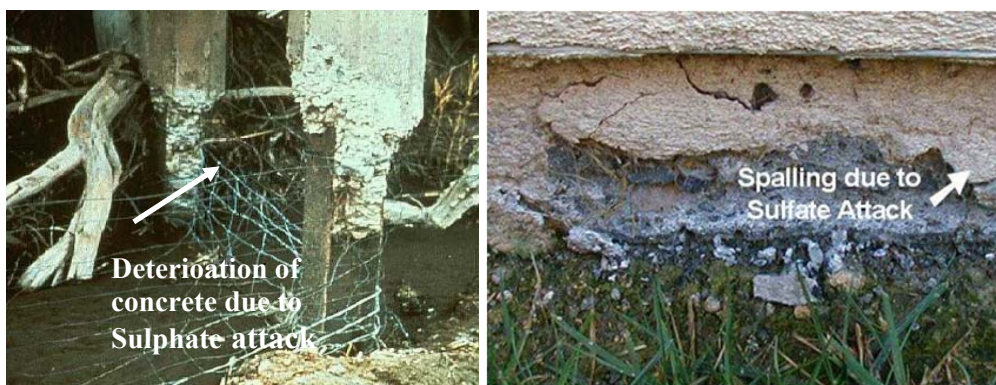
Figure 5.18. Deterioration in concrete due to sulphates [Collepardi 1999],
