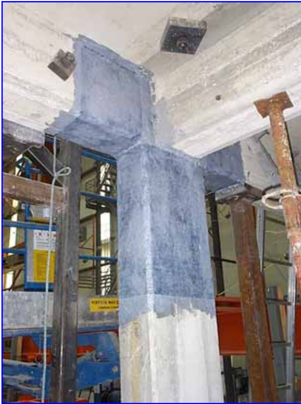
Figure 15. Reconstruction of the column/joint and strengthening with carbon fiber fabrics with epoxy based impregnation resin
