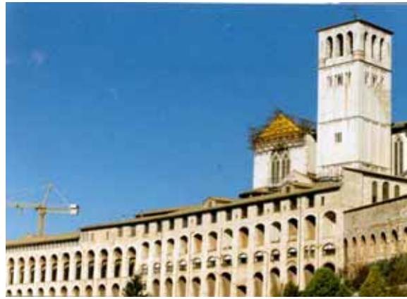
Figure 4. Repair and strengthening works at the Basilica of St Francis of Assisi (Tympanum) after the 1997 earthquakes, Italy
