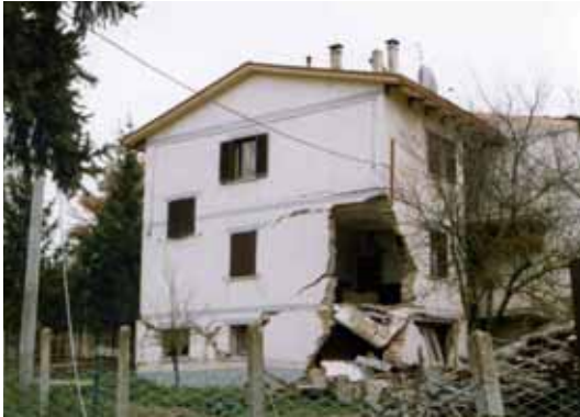
Figure 3. Failure (collapse of a corner) of a masonry house during the Umbria-Marche earthquakes, September 1997, Italy
