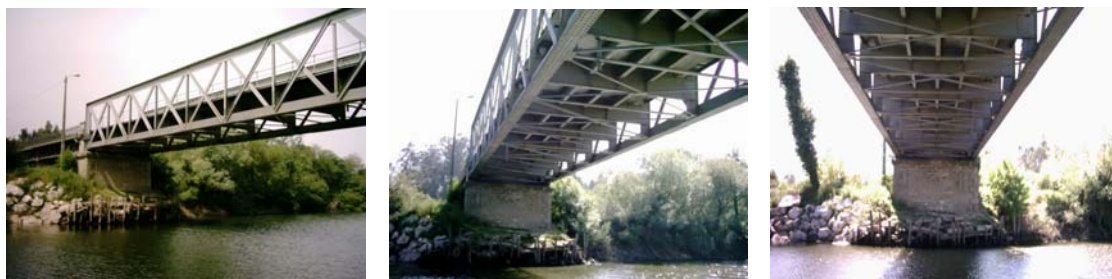
Fig. 1. General views of the S. João de Loure bridge (Fernandes and Silva 2004).
