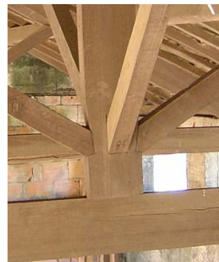
Fig 7 Example of a misconceived connection between the king post and the tie-beam
