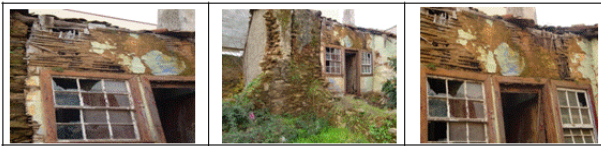
Fig.3 - Appraisal form filled for an example of a tabique construction existing in Macedo de Cavaleiros Municipality (November 2009)
