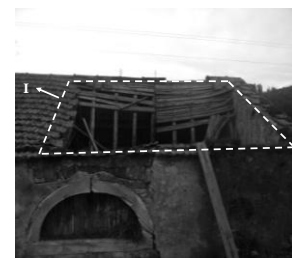
c. 3 rd Collapse (2009)
