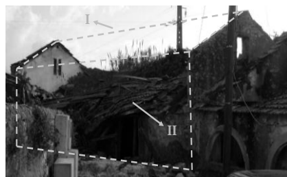
b. 2 nd Collapse (2007)
