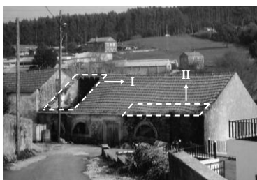
a. 1 st Collapse (2000)
