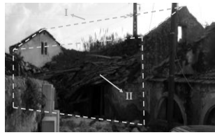
b. 2 nd Collapse (2007)
