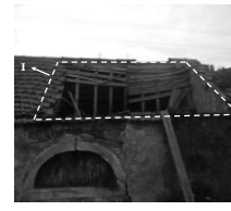
c. 3 rd Collapse (2009)
