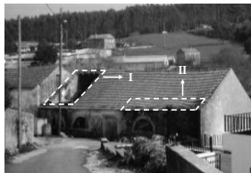
a. 1 st Collapse (2000)
