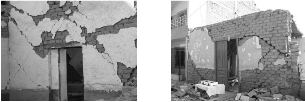
Figure 1. Failure of walls due to in-plane forces.
