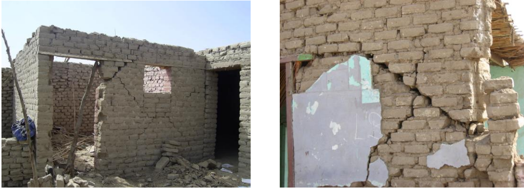
Figure 1.- Typical in-plane damage in adobe walls.
