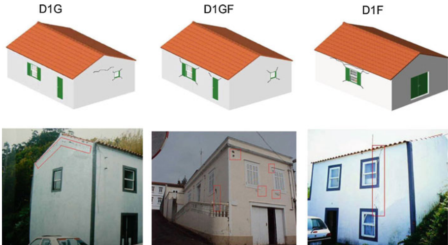
Fig. 7 Slight cracking damage examples (D1). D1G shows slight cracking in gable end wall, D1GF in gable end wall and front wall and D1F in front wall
