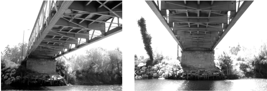
Figure 4. Bottom views of the S. João de Loure bridge: bracing system (Furtado et al., 2003)
