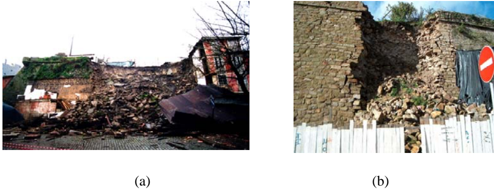
Figure 7. Scale of destruction of the SE wall of the Baluarte do Cavaleiro after the two collapses: a) First collapse (March 2001); b) Second collapse (April 2002)
