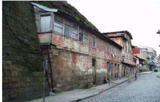
Figure 6. SE wall of the Baluarte do Cavaleiro and the existing attached buildings before March 2001
