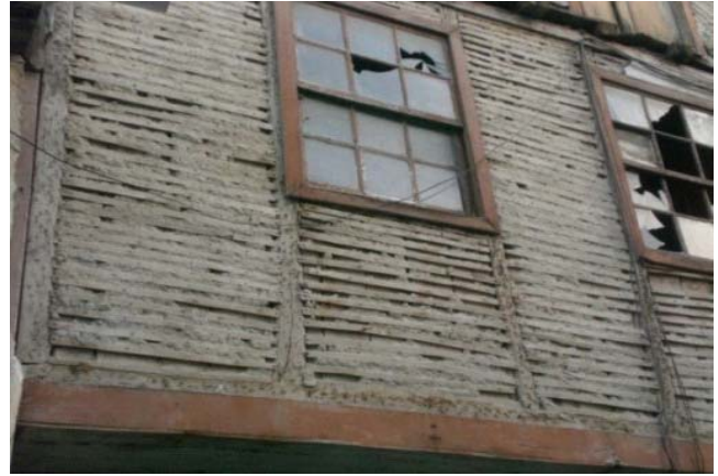
Fig.10 - Conservation state: Very deteriorated
