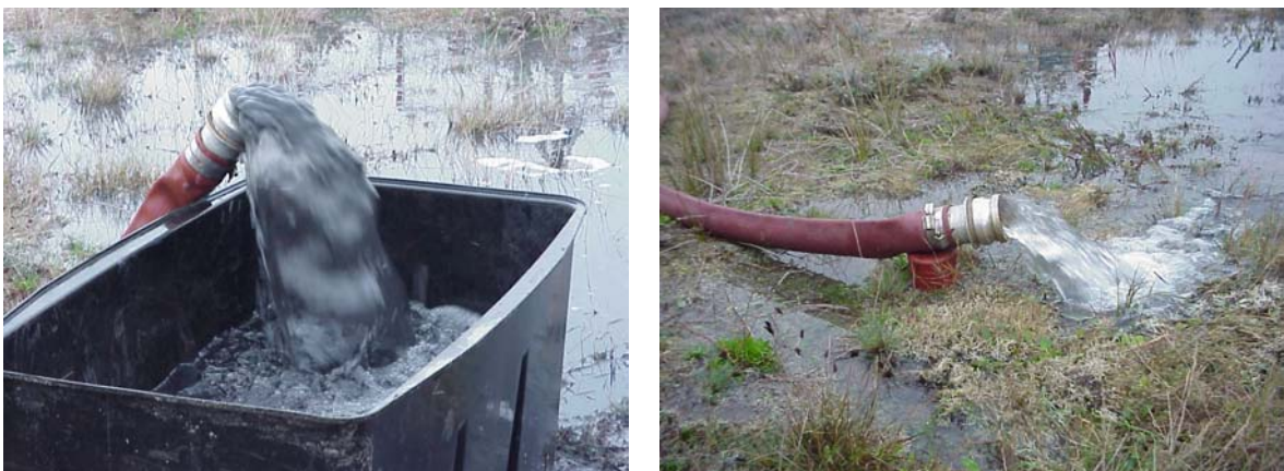
Fig. C.3 Borehole #11 (ACC01A Quintas do Sul) with the 100 mm diameter submersible pump installed to 24 m pumping a variable quantity of sand but able to gradually clear the borehole up to 128 m.
