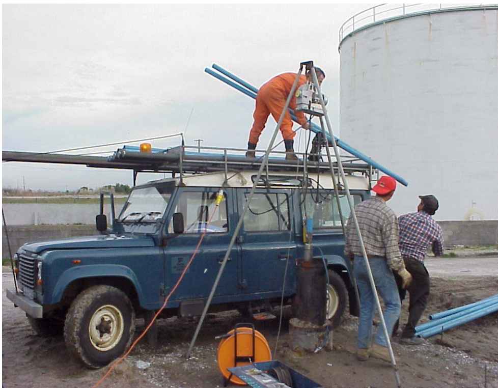
Fig. 5.24 Logger and tripod set up at borehole #62 (PS1 Gafanha da Nazaré). Also visible the electric hoist used to install the submersible pump and the pump itself.
