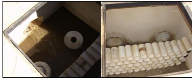
Figure 2. Junction box: entrance (left) exit and flow tranquilizer (right) (Silva et al., 2011)
