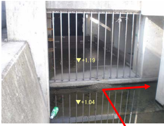
Photo 3-1 The Flow Intake (taken from ①)
