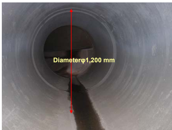
Photo 3-5 By-pass Pipeline (taken from ⑤)
