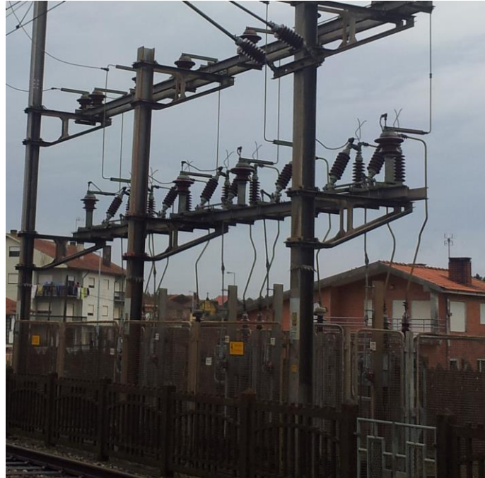
Figure 45: Outdated equipment at Ovar
