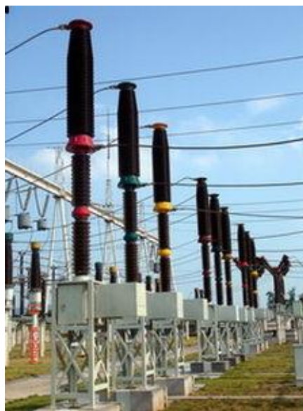
Figure 13:SF6 Circuit Breakers
