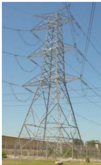
Figure 2: 400 kV double circuit strain tower
