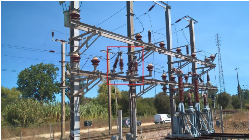
Figure 34: Switch (Seccionador) in Alfarelos Line
