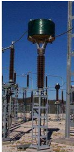
Figure 26: Filter consisting of a reactor and a capacitor
