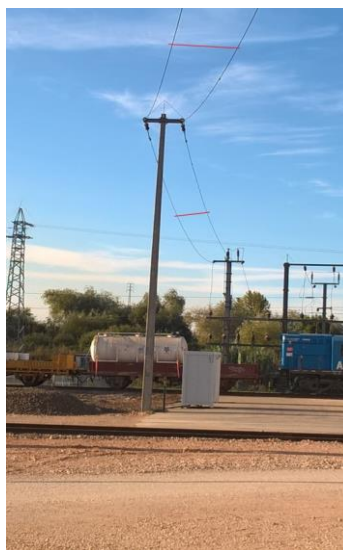
Figure 35: Aerial Feeder Lines
