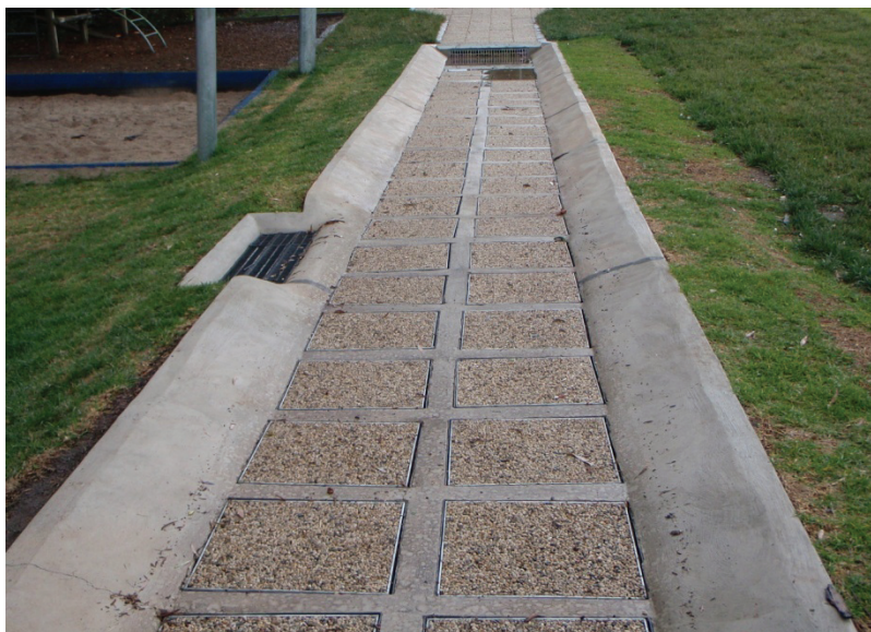
Figure 2: The stormwater treatment system at Syndal South Primary School.
