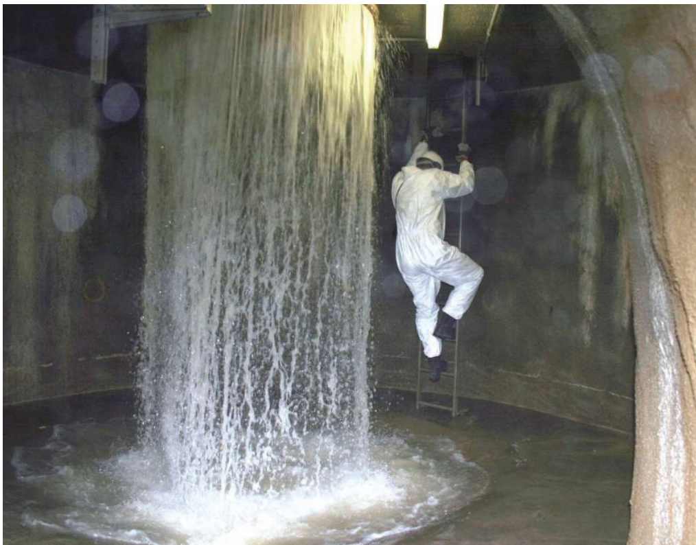
Fig. 8. Circular water jet falling down into the energy dissipation chamber of the Wiggen drop shaft during a minor rain event. The total drop head is 11.2 metres. (Photo: Hohl)
