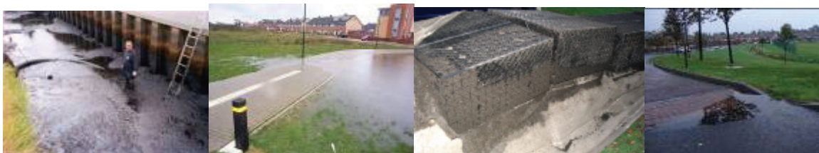
Figure 6 international educational SUDS: sediment load in stormwater basin, insufficient hydraulic capacity of swale, clogging of a infiltration system and bad construction of inflow.
