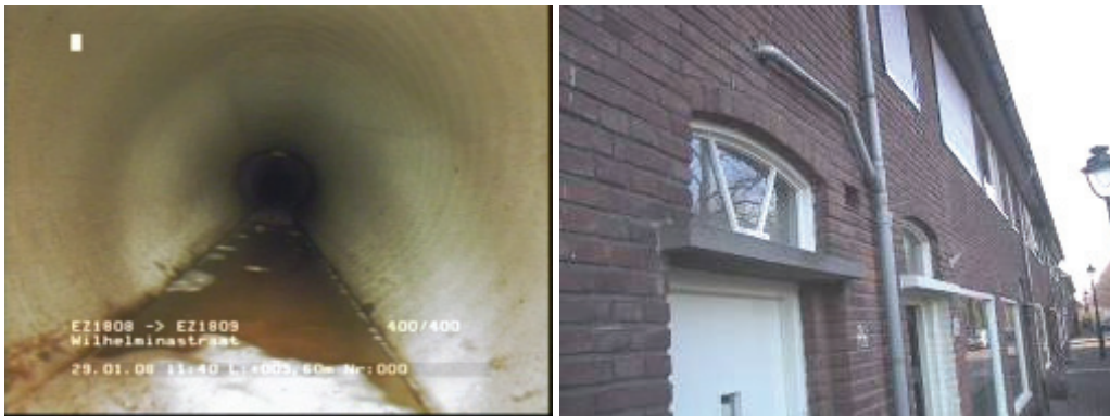
Figure 2: Stormwater drainage system with foul connections (left), connection of bathroom on a rainwaterpipe and stormwater drainage system (right).
