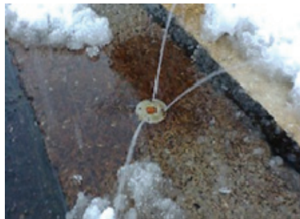
Figure 2 Sprinkling water from snow melting pipes in snowy season.
