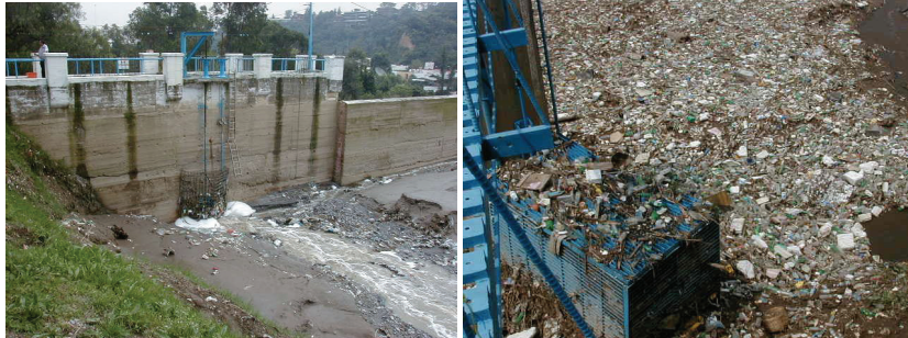
Figure 3. Sediment in El Capulin dam (left) and solid waste in La Colorada dam (right)
