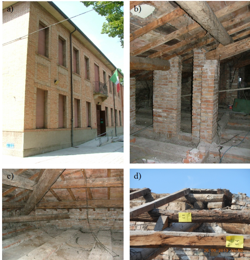
Figure 1: Some images concerning a building damaged by the Emilia Romagna earthquake of May 2012: a) An image of the building, b)-d) images of the timber roof elements.
