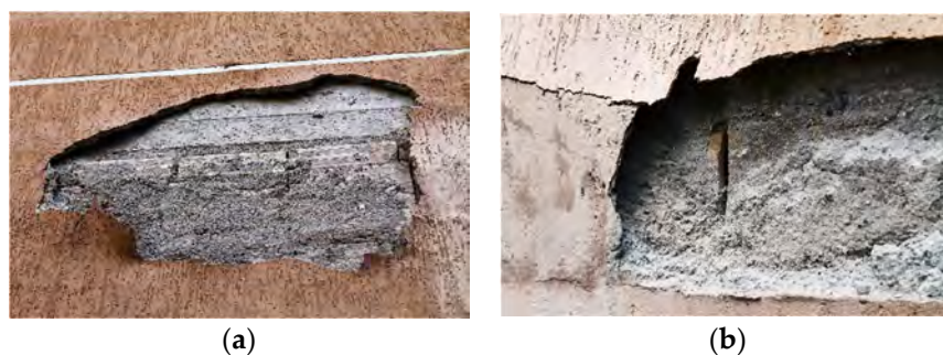
Figure 4. Hollow brick cavity wall: details with damaged plaster: (a) West façade, external wall below the reinforced concrete beam; (b) West façade, external wall in proximity to window sill.
