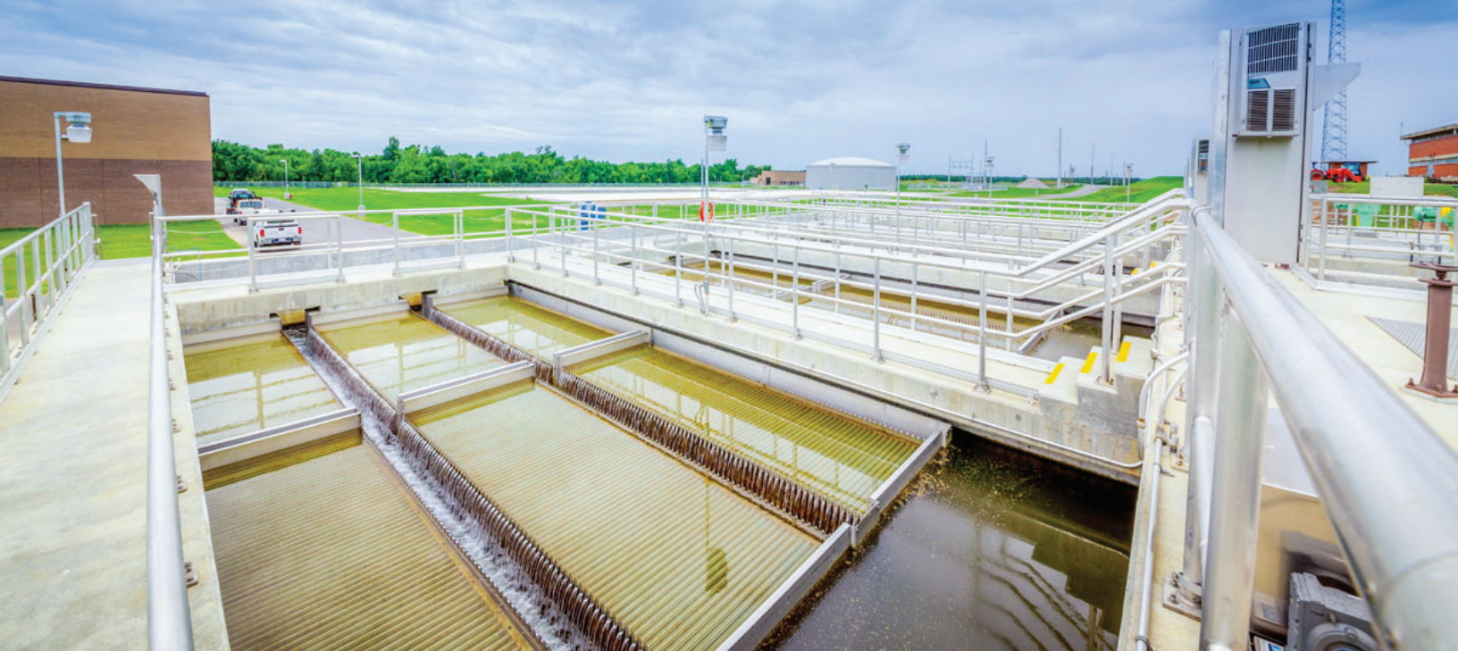
Image caption: Biofilm reactors at a wastewater treatment facility.
