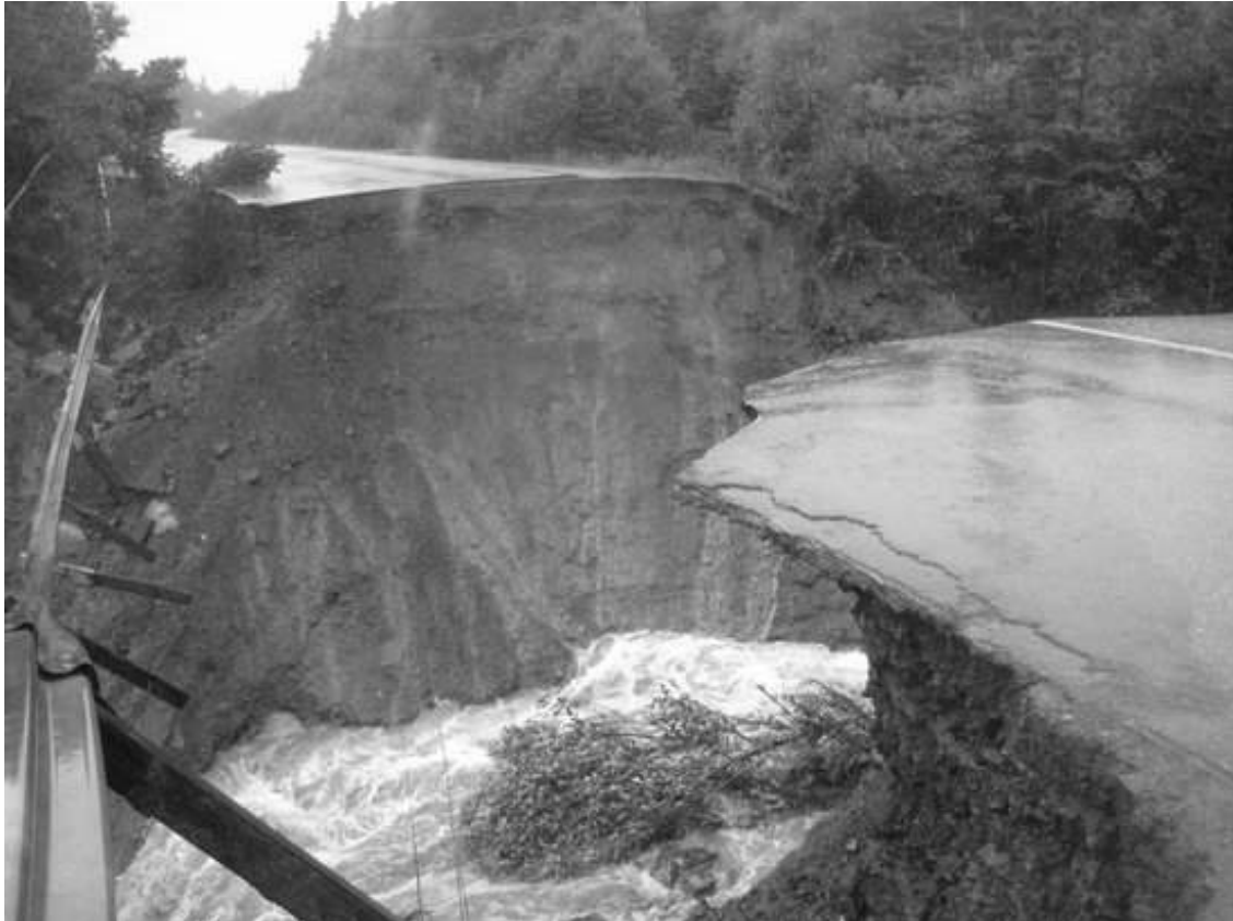
Photo 5.1: Typical example of type of damage to roadway caused by Hurricane Igor - Little Barasway, Avalon Peninsula (Rose 2010)
