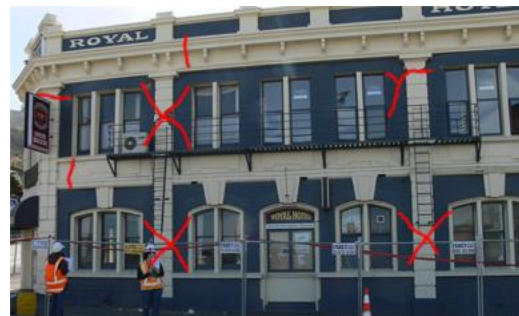
b) Façade of RH on Norwich Quay. Cracks are highlighted in red for clarity
