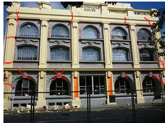
b) East façade of AH after the earthquake. Damage was mainly in the spandrels and external piers
