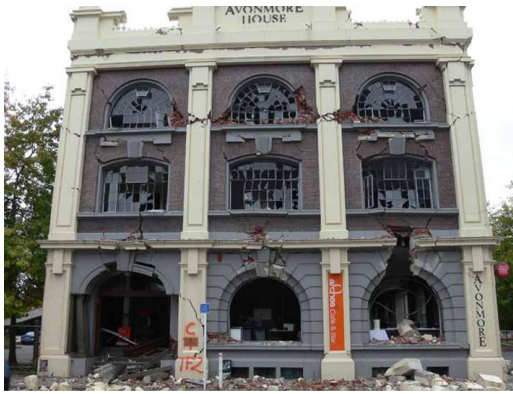
a) South façade of AH after the earthquake. Damage is evident in the spandrels and in the exterior and top piers
