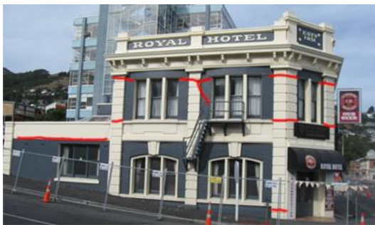
a) Façade of RH on Canterbury road. Cracks are highlighted in red for clarity
