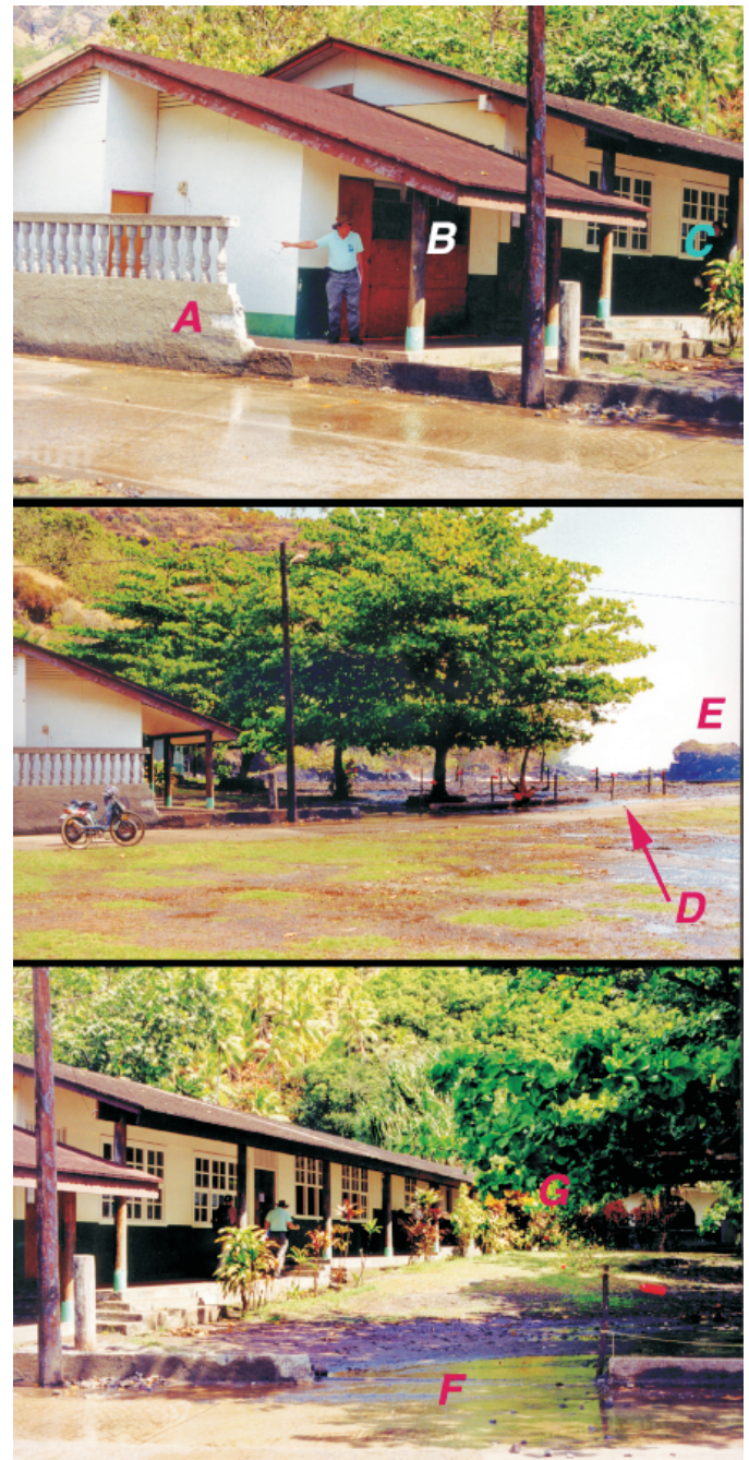
FIG. 3. – The damaged school at Omoa, photographed on 4 October 1999. Top (looking SSE) : The wall (A) has been totally destroyed around the playground. The principal's office and teachers' room (B) have been damaged and are now boarded up. Classrooms located at slightly higher elevations (C) were merely flooded. Center (looking SW) : The wall (A) used to extend all around the yard (to point D), and has been destroyed. Note the Motutapu promontory in the distance (E), which provided some protection to the southern part of the bay. Bottom (looking south) : (F) shows the location of the entrance gate through the wall. Note the slight incline to the south which lessened the impact of the waves on the more distant classrooms, and especially on the pre-school building (G; hidden behind shrubbery).
