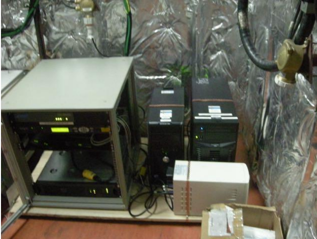
Image 4.6. The server room of the Victorious, located just below the Wheelhouse. (Image slightly blurry due to moving vessel). Photo: Aug. 17, 2010.
