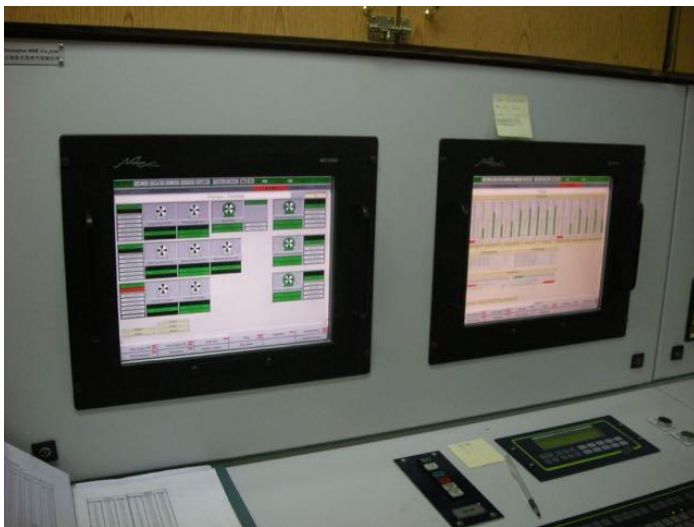
Image 5.3. The NORIS screens in the engine control room on the Victorious. These displays allow engineers to monitor pumps, levels, equipment functionality and more. Photo: August 12, 2010.
