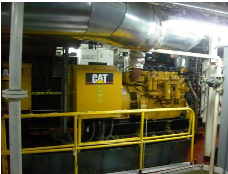
Image 6.6 One of the generators in the engine room of the Victorious. Photo: August 11, 2010.
