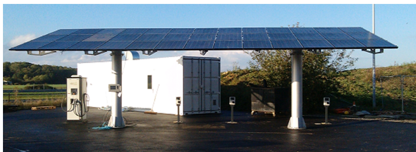
Figure 3.6: EVEREST project platform in the U.K., with a container where batteries and electronic equipment will be installed and the solar carport and EV chargers
