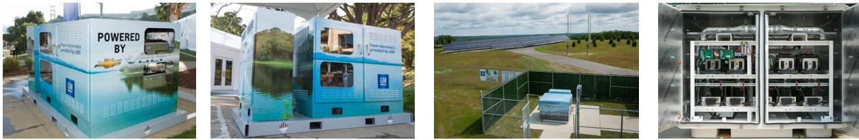
Figure 3.4: First and second ABB-GM energy storage demonstrators projects in the US. The two images on the left correspond to the 1 st project, the images on the right to the 2 nd .
