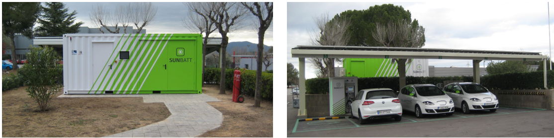
Figure 3.10: Sunbatt project demonstrator at SEAT facilities in Martorell, Catalunya, Spain. Left: Entrance to the container where batteries are stored. Right: Rest of the installation, with the solar panels, the chargers and the container in the back.
